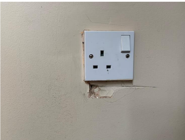
Firestopping repairs required
