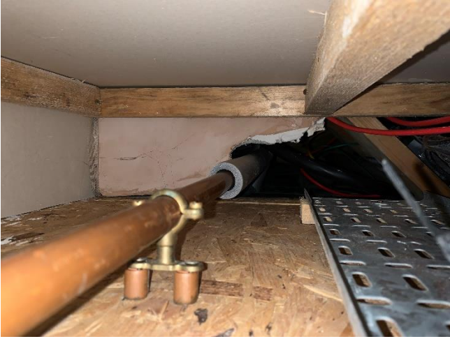
Firestopping improvements required
