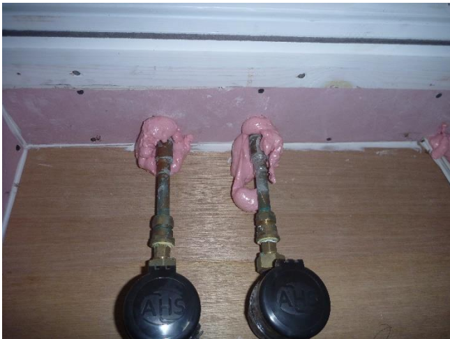
Inappropriate use of foam
