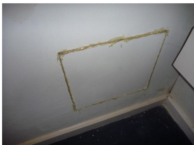
Ensure long-term repairs provide acceptable fire resistance
