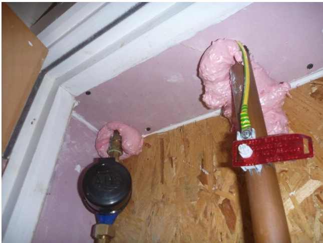
Excessive use of foam
