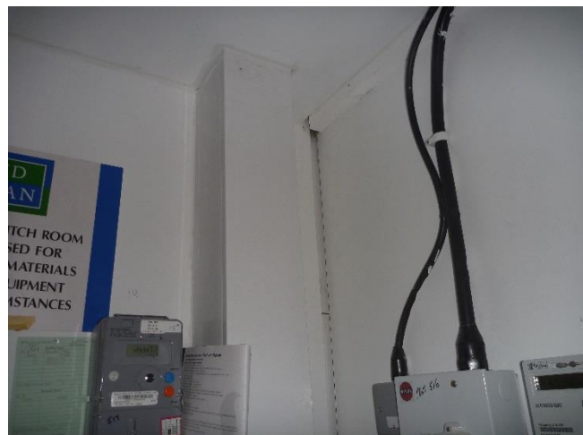
Firestopping improvements required
