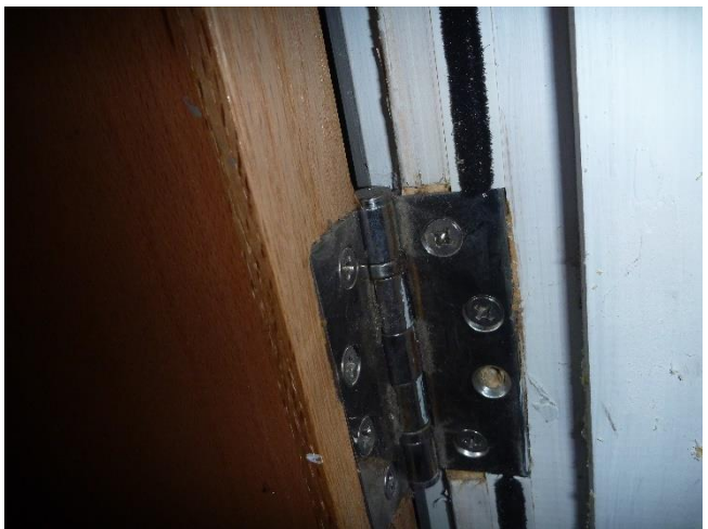
Missing hinge screws
