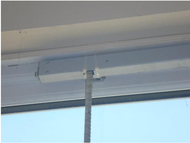
Damaged AOV mechanism
