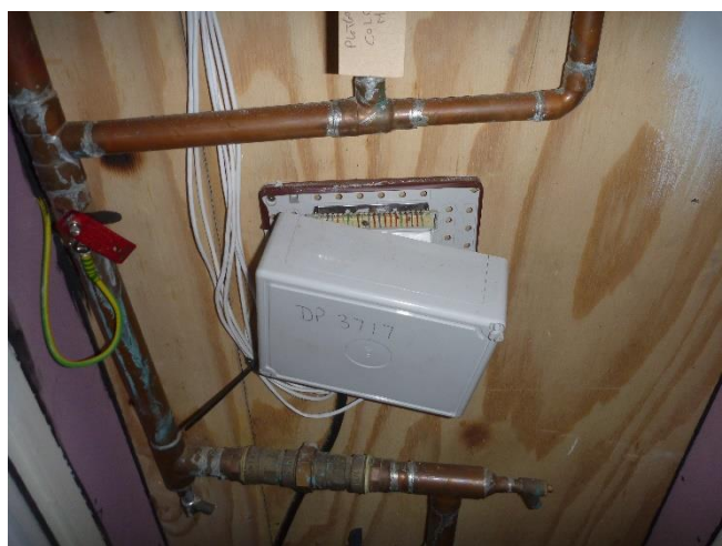
Telecoms box cover loose
